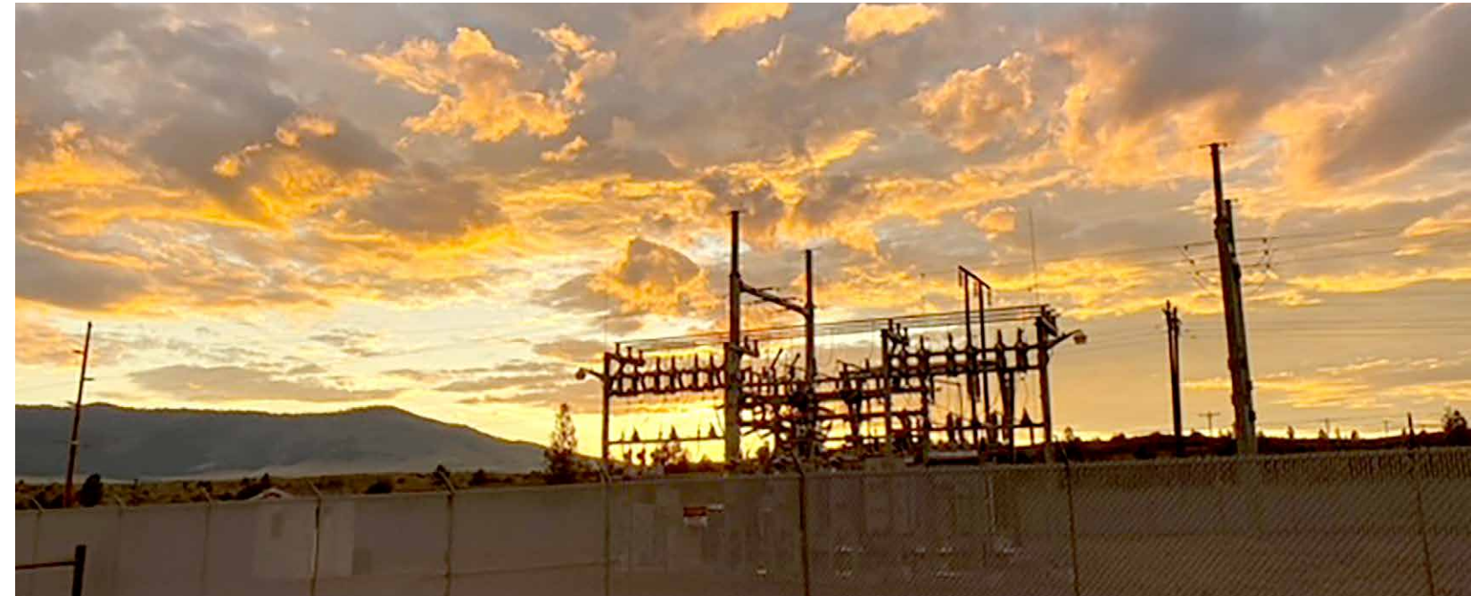
MVP distribution substation located at Irvine.
